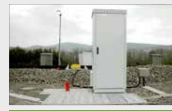
Axle counter, zone controller, wheel T°, track maintenance, interlocking.
