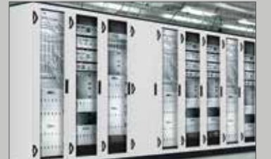
Signalling & Passenger information systems
